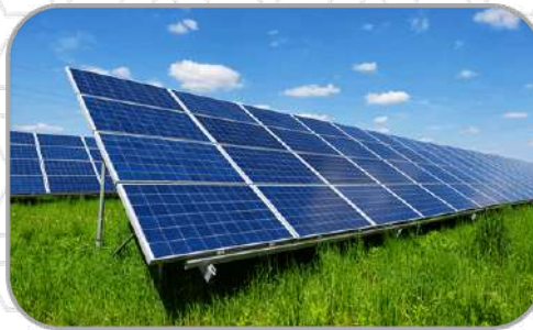
INDIA'S LARGEST 5000MW SOLAR PARK
