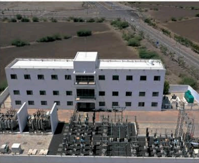
Power Substations 2 Substations (33/66 Kv and 220 Kv GIS) by Torrent Power
